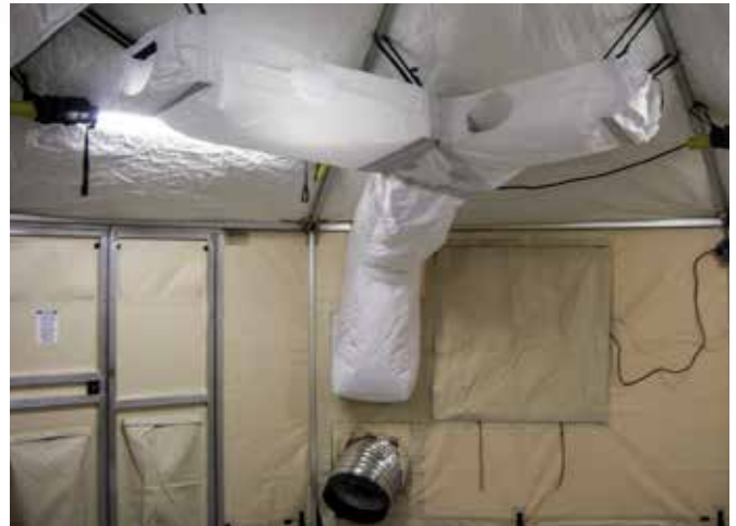
CL-20AP hanging in SW-20 shelter
